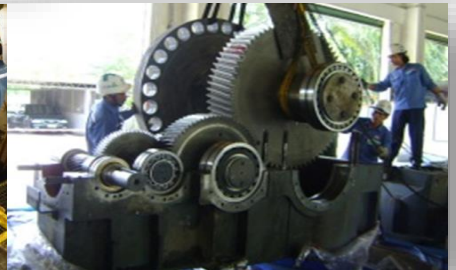
Gear box Overhaul
