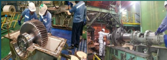
Manage and Supply Mechanical Skilled Manpower-TCRSS
